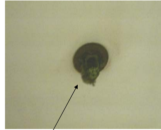
Dirty sprinkler head
